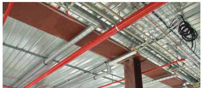
Figure 3.3 Built-in under floor technical equipment (Petrusse Building, Luxembourg)
